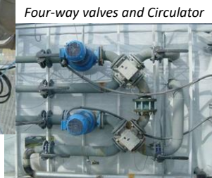
Four-way valves and Circulator
